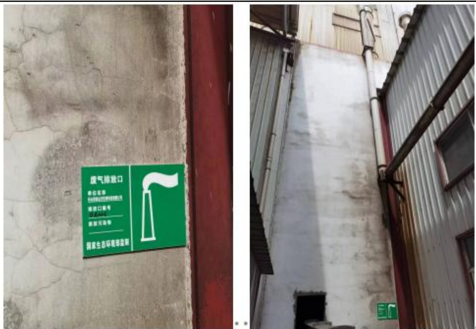
DA006 ····· DA006 废气治理设备
