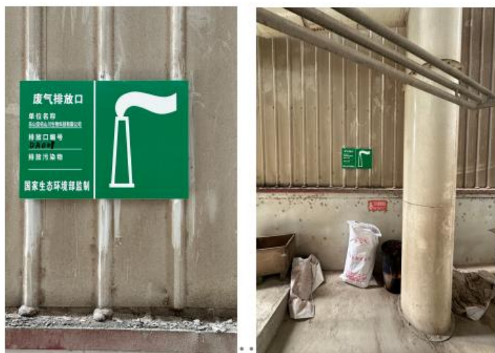
DA001·····DA001 废气治理设备
