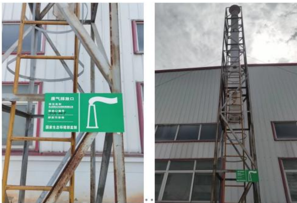
DA007 ····· DA007 废气治理设备
